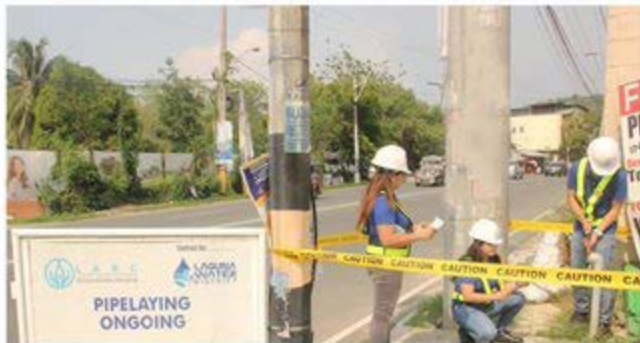
Pipelaying Project. LARC employees conduct final inspection of hydrant at Lalakay, Los Baños to check water pressure after the project completion on February 2019.
